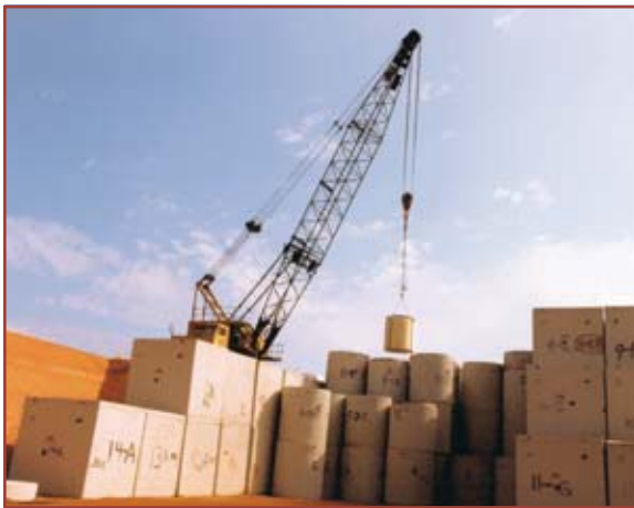
High Integrity Container of Class A LLRW being placed in a cylindrical disposal vault.
