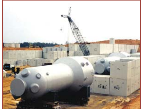
Low activity commercial reactor steam generators placed among disposal vaults for burial.
